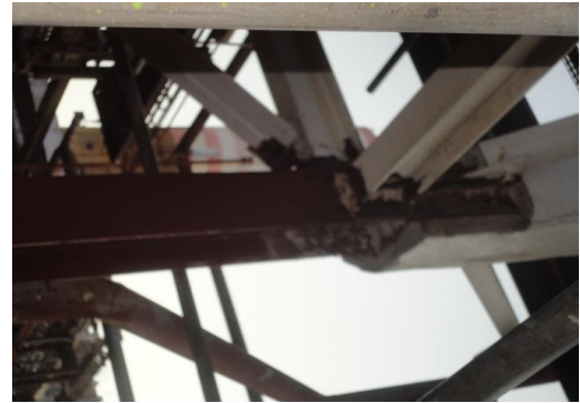
Gambar 1. Korosi dibawah fire proofing (Corrosion under fier proofing)
